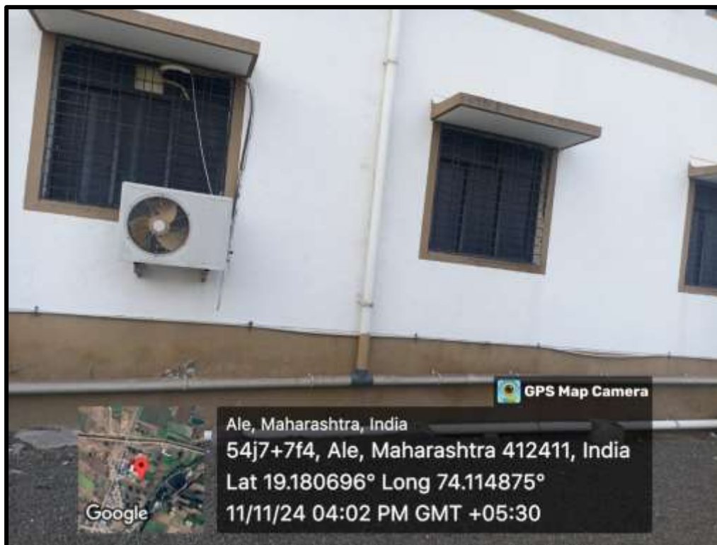
Collection of rain water through centralised pipe line
