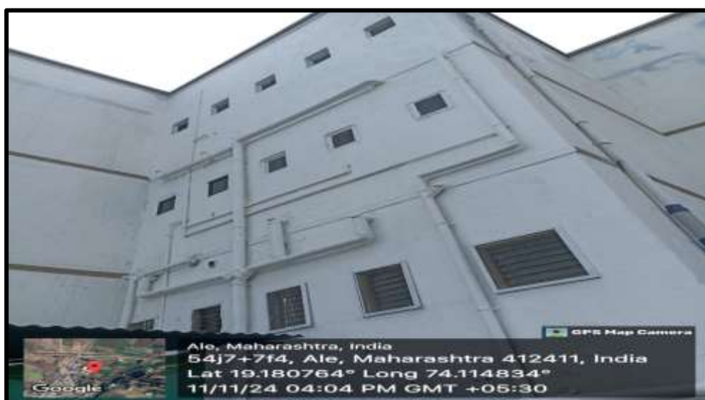
Distribution channel of water through centralised tanks
