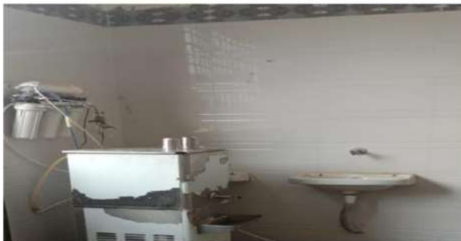
R.O. System installed in college
