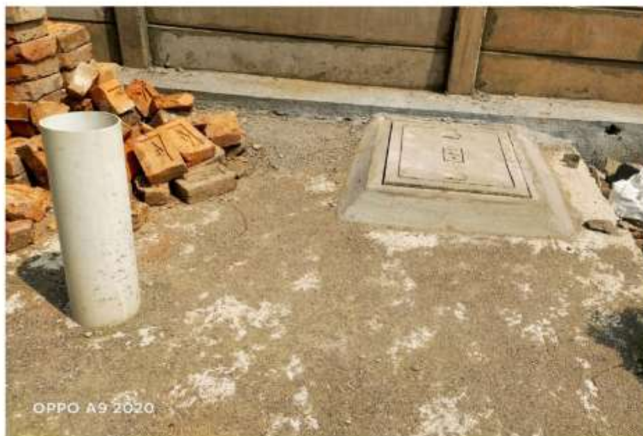
Rain water Harvesting Recharge Tube
